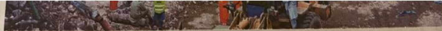
THE use of heavy machinery for debris removal has sparked fears of desecration of the remains of Gul Plaza fire victims.—Shakil Adil / White Star
